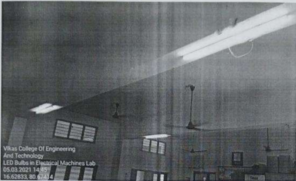
LED Bulbs at Electrical Machine Lab
