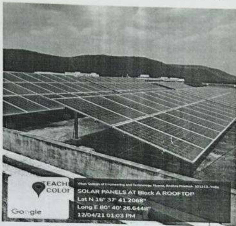
Solar Power panels at Block-A Roof Top
