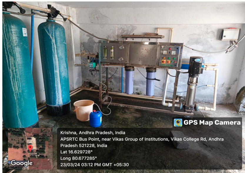
RO Water plant
