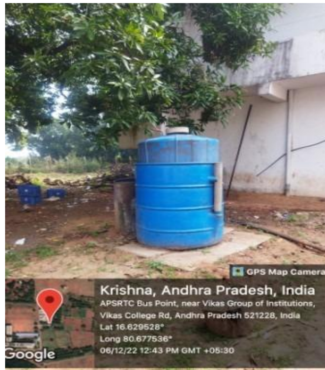
Bio Gas plant
