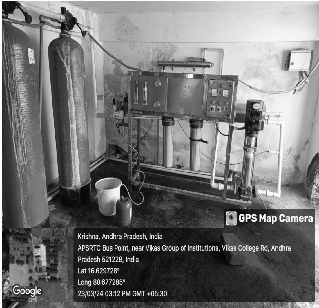
RO Water plant
